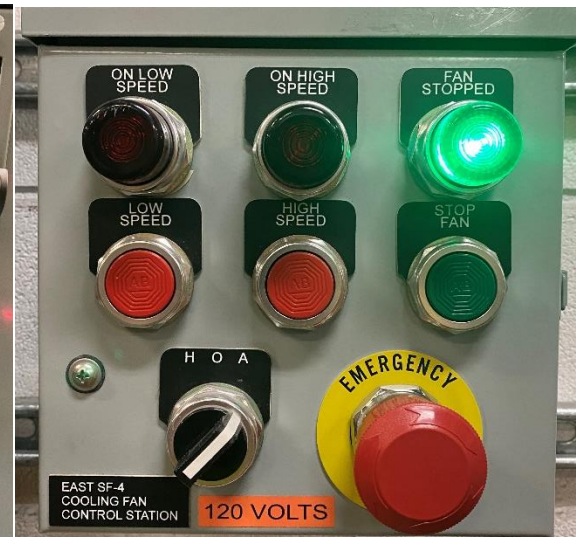
Local Control Station
