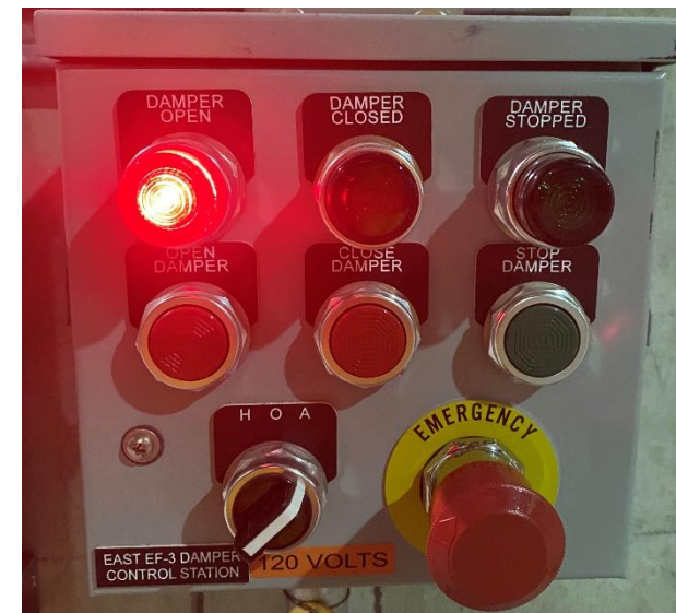
Local Control Station
